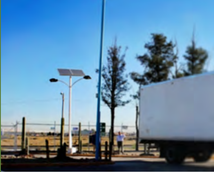
Flextronics Aguascalientes, Mexico | Solar Panels
